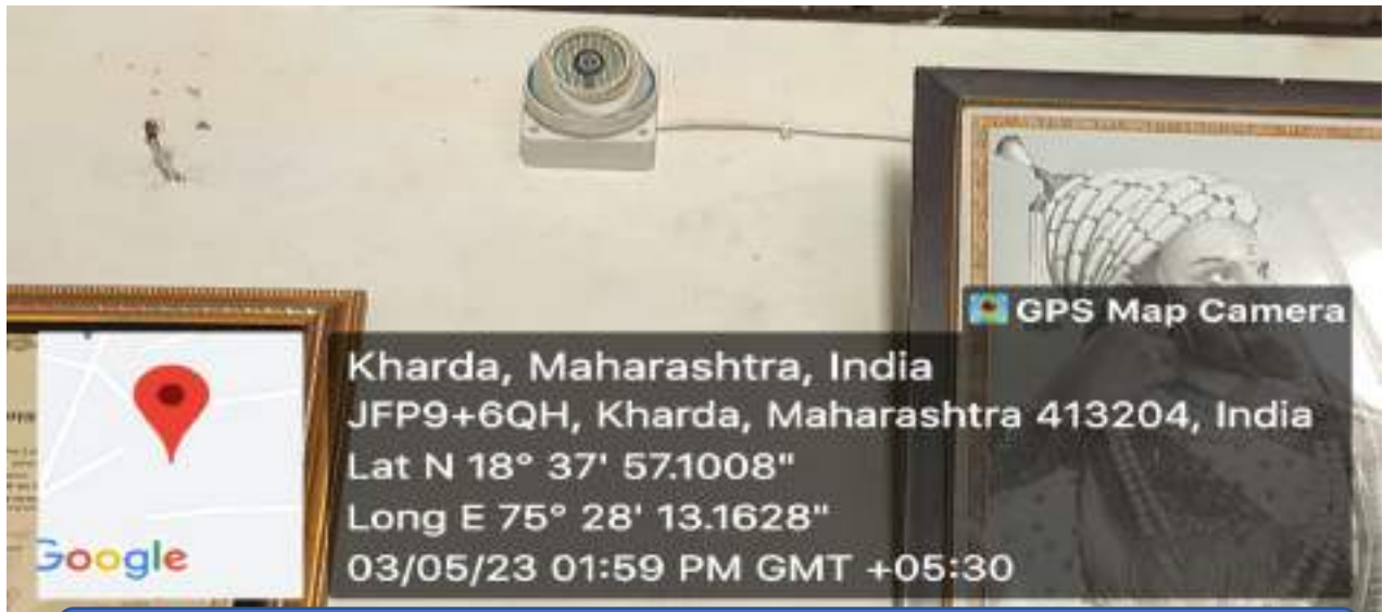
CCTV Under Principal Cabin
